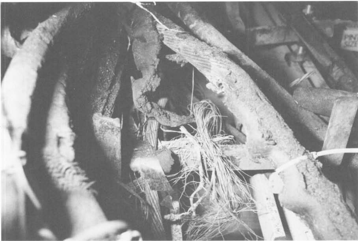
Photograph 3-45. 750 MCM power cable and stanchion; both damaged by arcing between them, Section 1, F cut.
