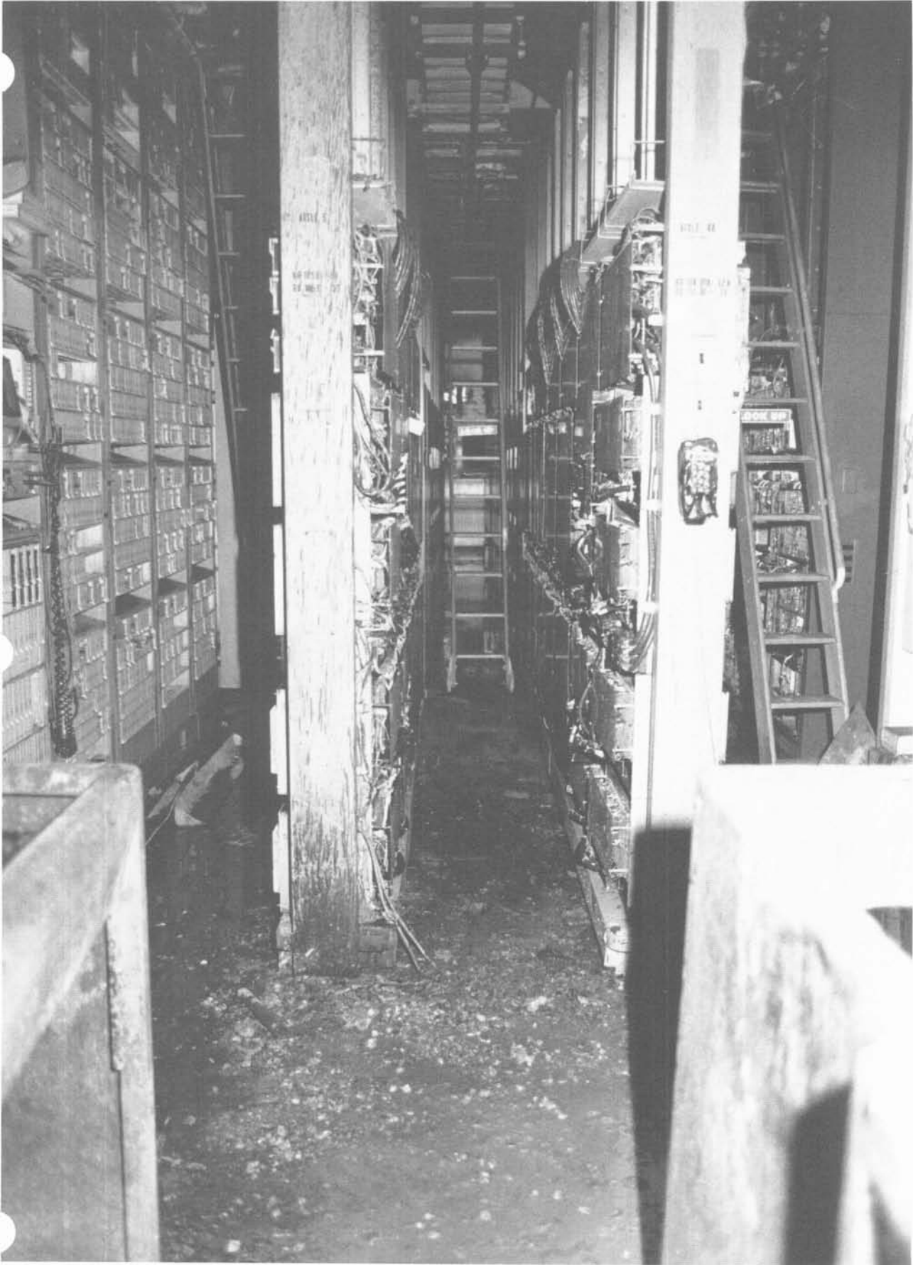
Photograph 3. Fire damage below cable trays shown in Photograph 2.
