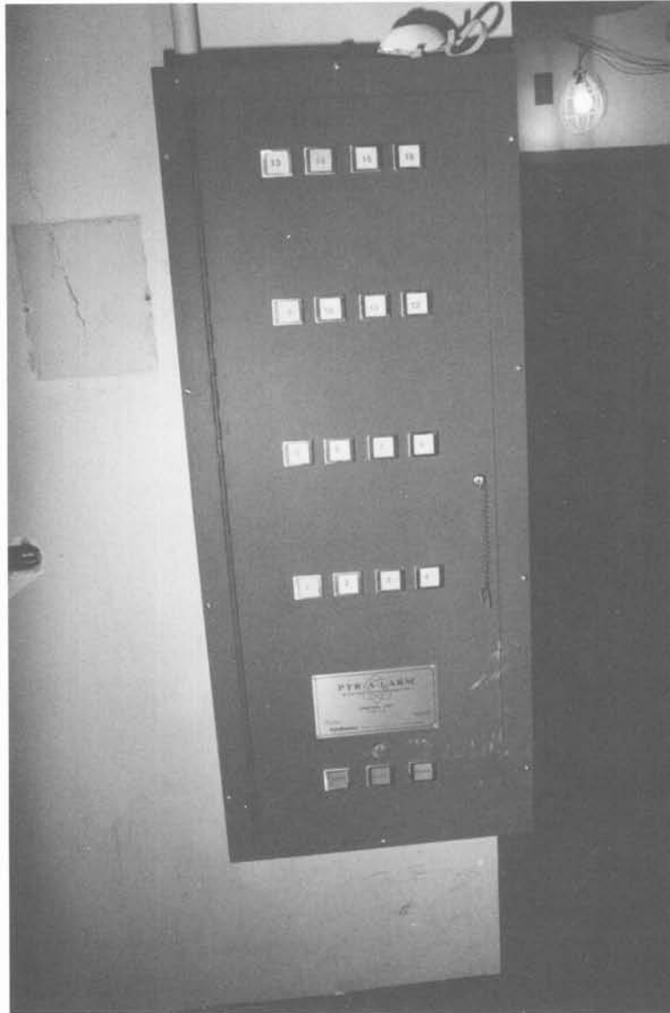
Photograph 3-26. Pyrotronics fire alarm annunciator panel on the first floor.
