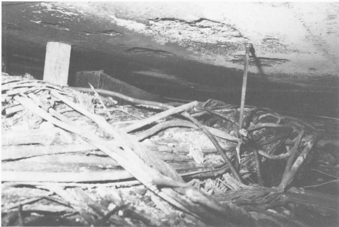
Photograph 3-20. Spalling of concrete above arced cables in cable trays, Section 2.
