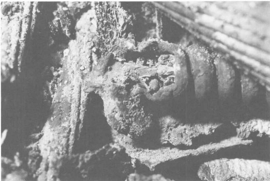
Photograph 3-15. Armored cable welded to a 4/0 power cable in Section 1, near L cut.
