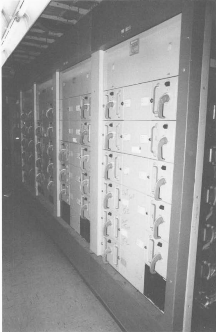
Photograph 3-33. 326 power supply fused discharge bay in basement.
