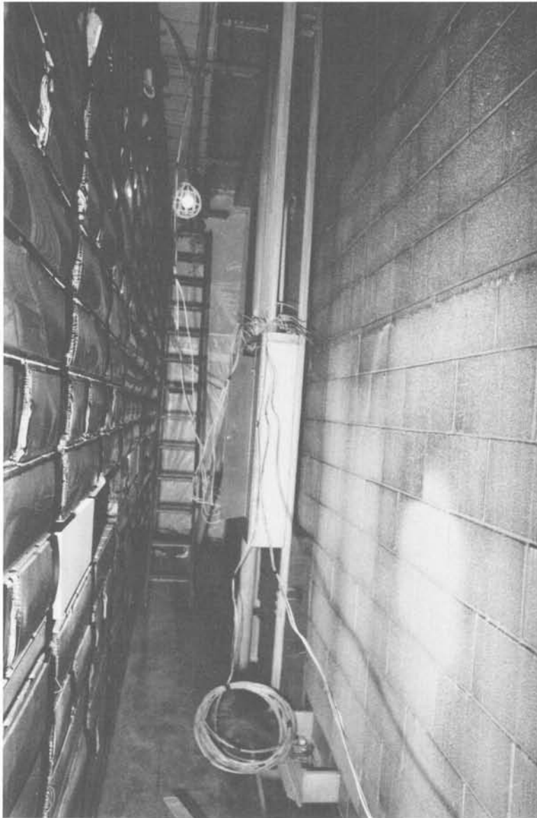
Photograph 3-25. Smoke damage in northwest corner of toll area, first floor. (North wall.)
